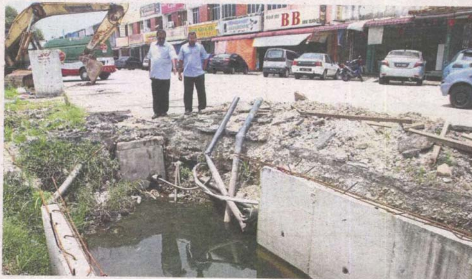
Parts of Taman Sentosa, Klang, dug up for a flood mitigation project, are still in a mess.
